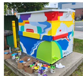
Painted padmount transformer box on the corner of Harbour Drive and Water Street, St. John’s.
